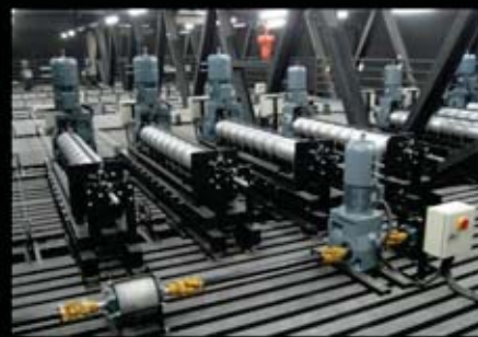
Fly-bar Machinery & Bar Hoist
