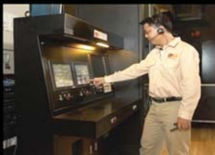
Computer Control System
